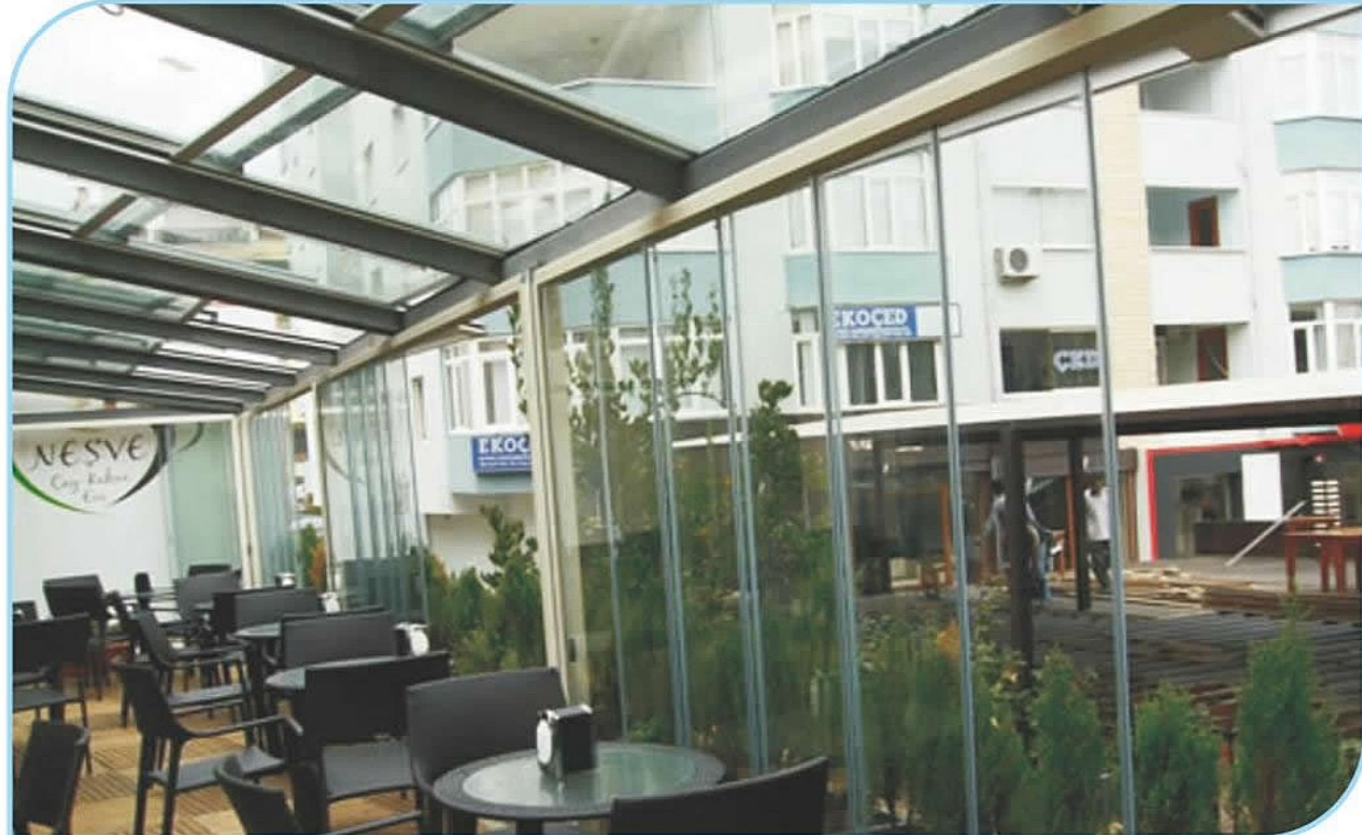
WINTER GARDEN WITH SUNROOF GLASS CEILING AND 8 MM TEMPERED AND WITH EDGING FOLDING GLASS APPLICATION
